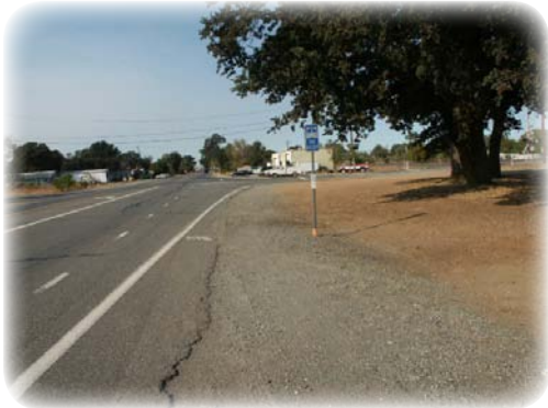
The lack of an accessible path makes it difficult for a wheelchair user to use this stop in Red Bluff, California. All users would have to travel on gravel and on the roadway shoulder to use the stop.
