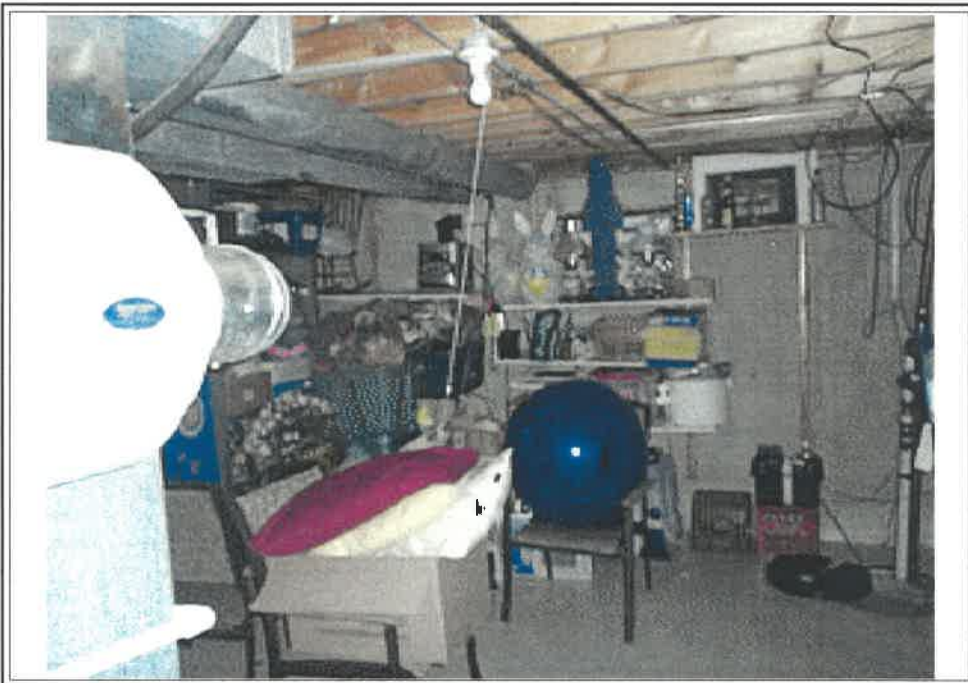
Basement storage, note humidifer attached to furnace on left side foreground of photo.
