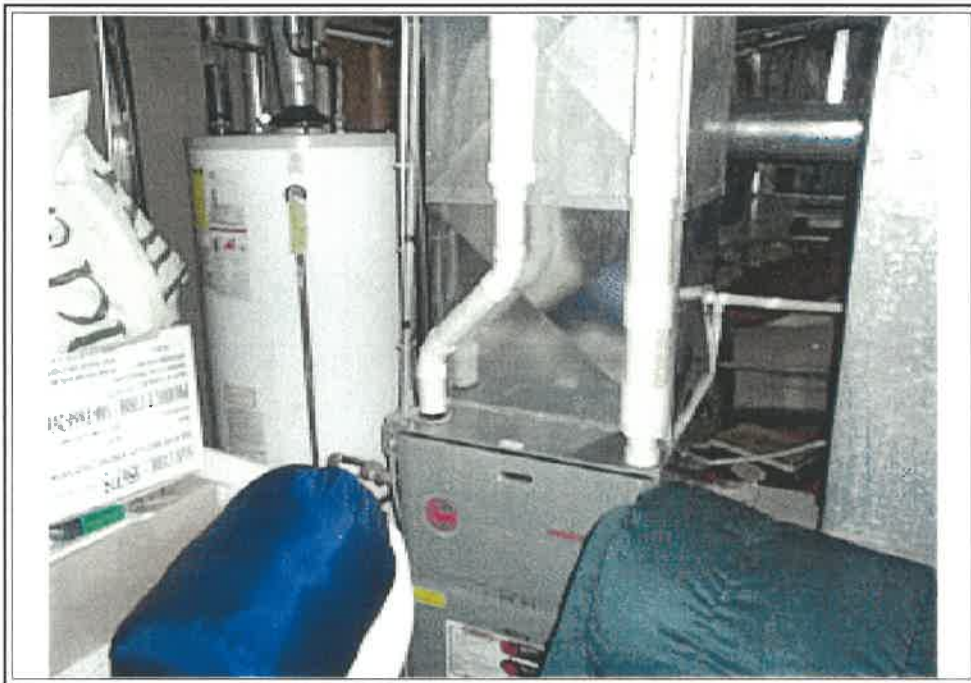
Gas fired forced air furnace replaced in 2003 along with 75 gallon gas fired hot water tank. Owners added humidifier.
