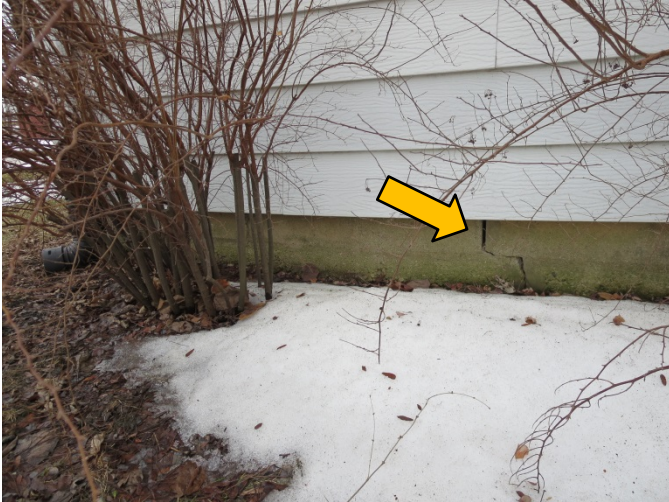
Photograph 6 Detail of concrete block foundation at east end of north facade. Note open mortar joints.
