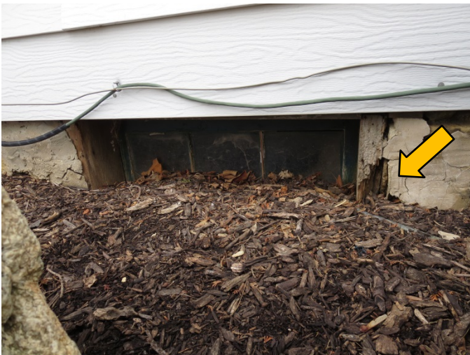
Photograph 21 Detail of basement window at south facade showing dirt mounded above the window sill. Note deterioration of exposed wood framing at window.
