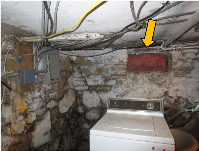
Photograph 4 Interior view of basement showing stone foundation wall. Note window blocked by insulation.
